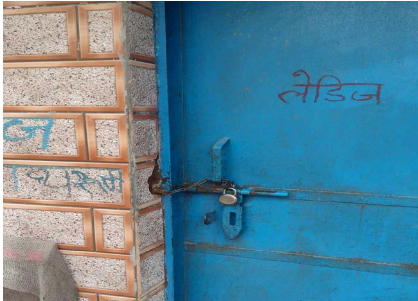
Image 8: The locked public washroom supported by an NGO in Kalkaji Market
