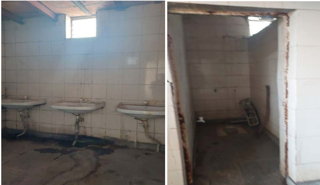
Images 9 and 10: These images depict the dilapidated condition of the ladies' washroom in Daryaganj Sunday Book Market.
